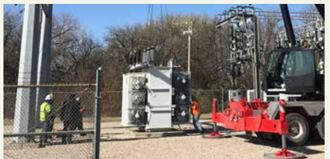
New Andale substation transformer installed to provide projected increase demand usage.
