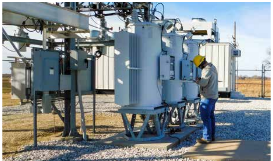
Apprentice Lineman Tommy Hill conducts a monthly substation inspection.
