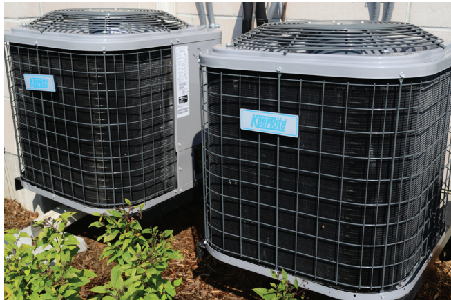
Tracking energy use and maintaining the heating and cooling system can help small business owners save on energy bills.
