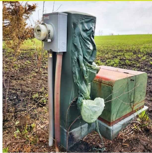
Before burning, check the property for electrical equipment — like this pad-mounted transformer — and power poles to avoid damage and potential outages.
