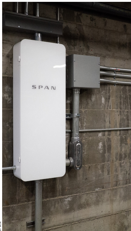
With smart breaker boxes, like the SPAN Panel shown here, you can control and monitor every circuit in your home from a smartphone or tablet.
